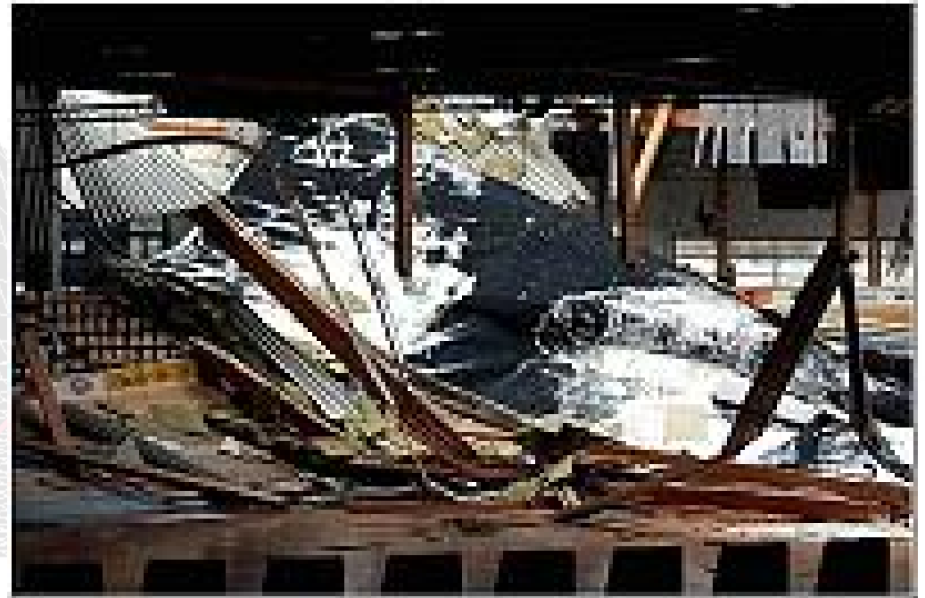
Design/execution errors Siemens Arena
