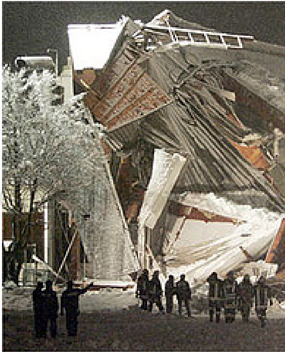
Extreme loads/deterioration Bad Reichenhaller
